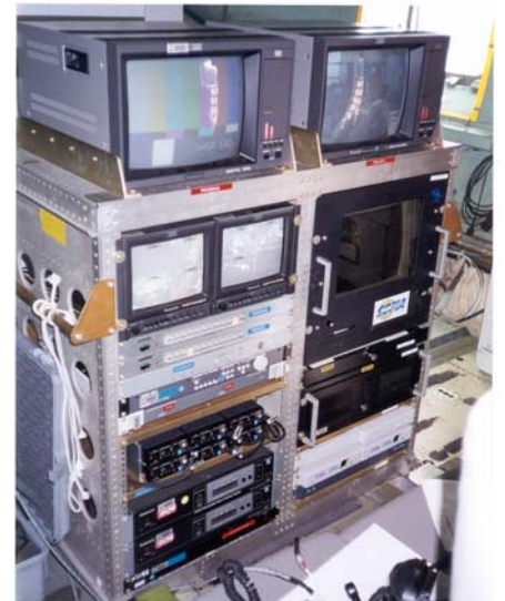
The left bay contains all the video equipment and the right side contains the ACTS antenna tracking computer and audio equipment.
